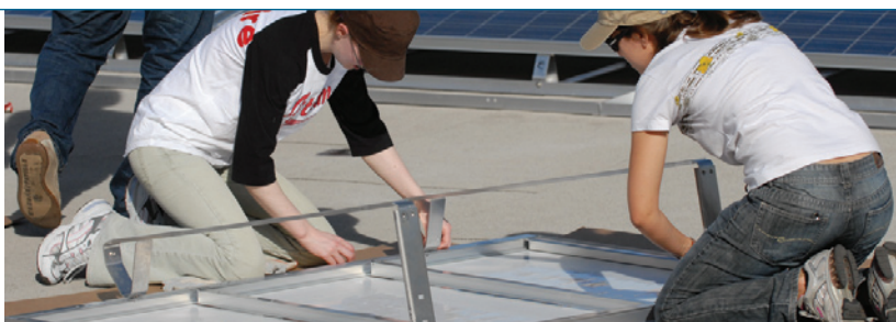
Atwater postdocs Dierdre O'Carroll and Marina Leite install the support structure on the back of a solar panel.
